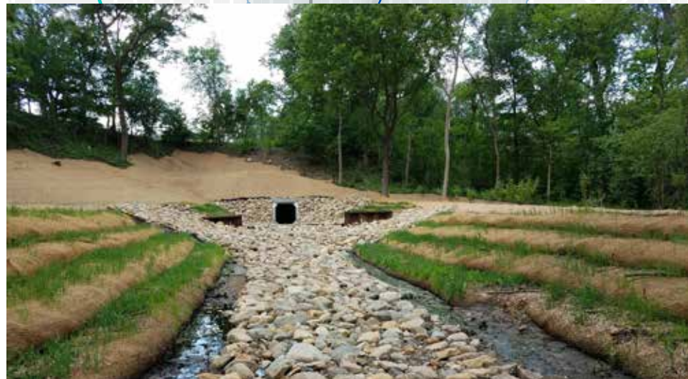
Energy dissipation basin is used to reduce the water's energy at Lyndale Avenue
